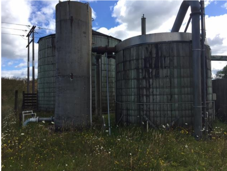
Figure 7: Tihiroa Contact Tank, Clarifier and Filter
