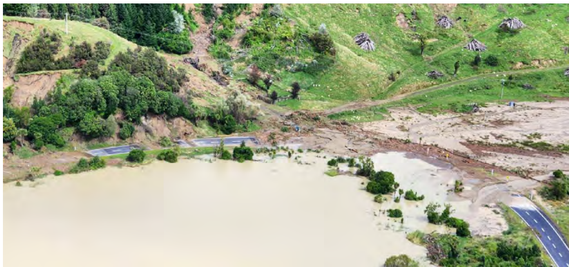
Image: A section of SH2 between Napier and Wairoa was washed out. Source: NZTA
