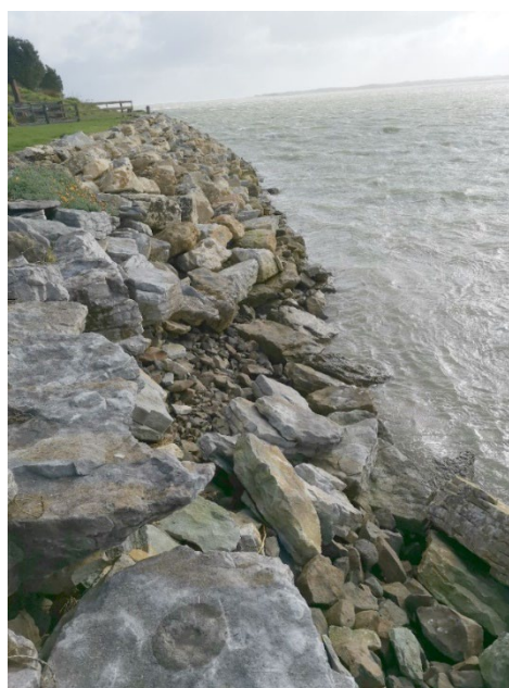
Slumping and loss of rock armour ch. 250 – 350m
