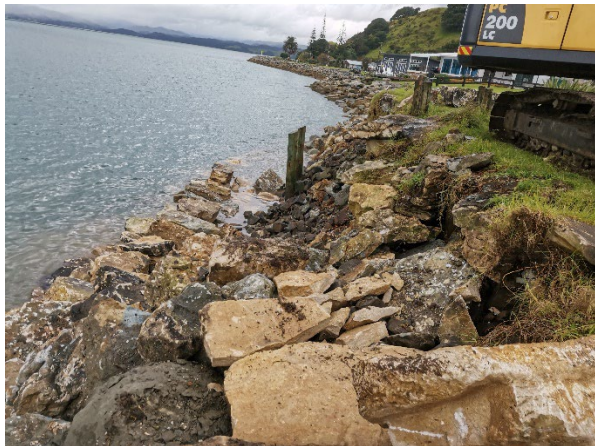
August slump zone
