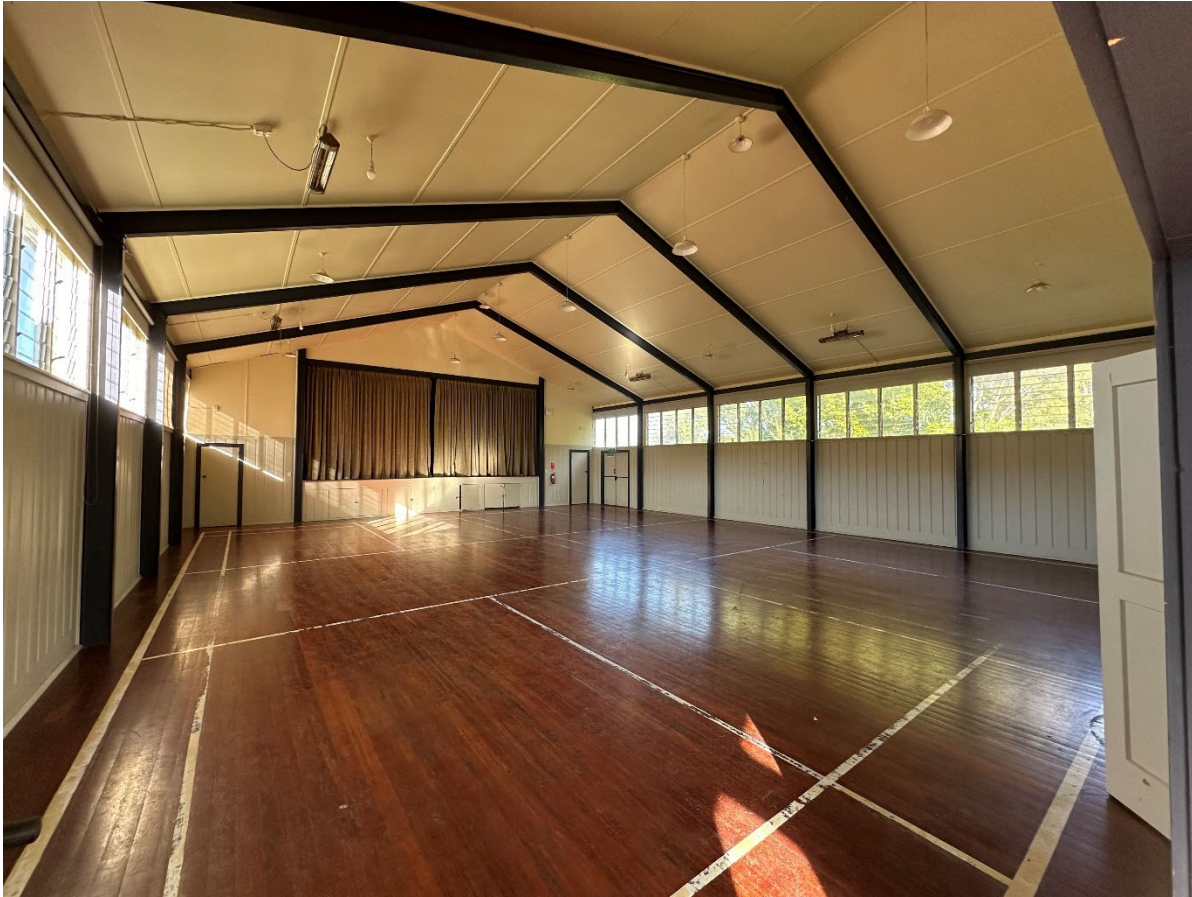
Internal Hall area showing steel portal frames and eaves tie-beams with timber sub-floor structure.
